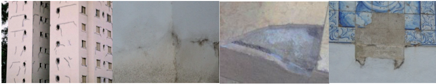
Figure 19. Different types of materials applied as façade coatings and some irregularities.
