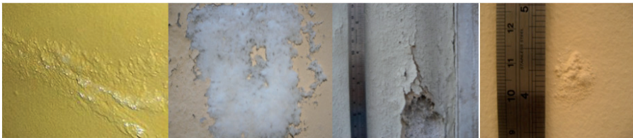
Figure 11. Swelling, efflorescence, cracking and blistering (Moura. 2008).
